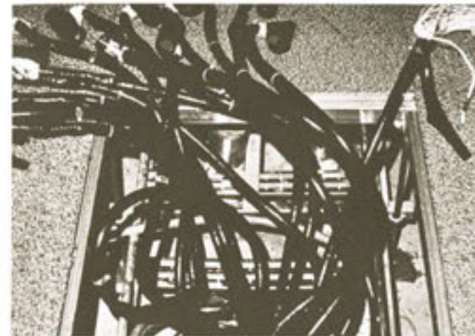
FIGURE 15: Control Room cable terminations.
