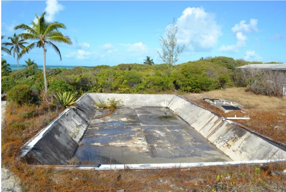
Photo 4-58. Abandoned Concrete-Lined Water Storage Structure adjacent to Former Staff Housing on Children's Bay Cay
