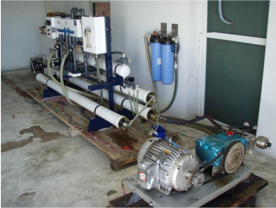
Photo 4-56. Reverse Osmosis Plant
