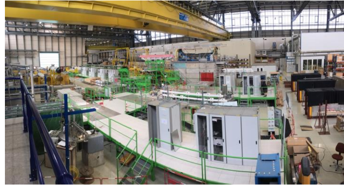
CERN: Test facility completed for the Super-FRS s.c. dipoles and multipllets
