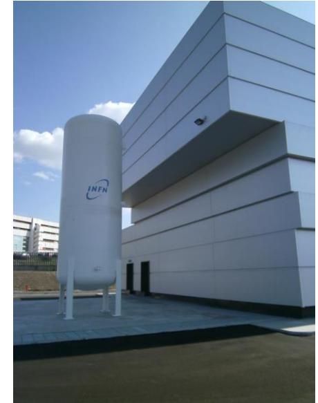
INFN: Test facility in Salerno for testing the series of SIS100 quadrupole modules
