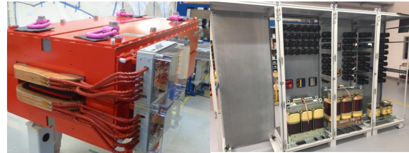
Bipolar dipole magnet and power converter for the connection of transfer line to SIS100
