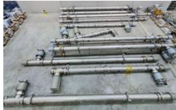
Bypass lines in storage area Weiterstadt
