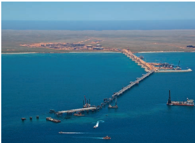
The Materials Offloading Facility and LNG Jetty in construction on the east coast of Barrow Island. Photo - Chevron
