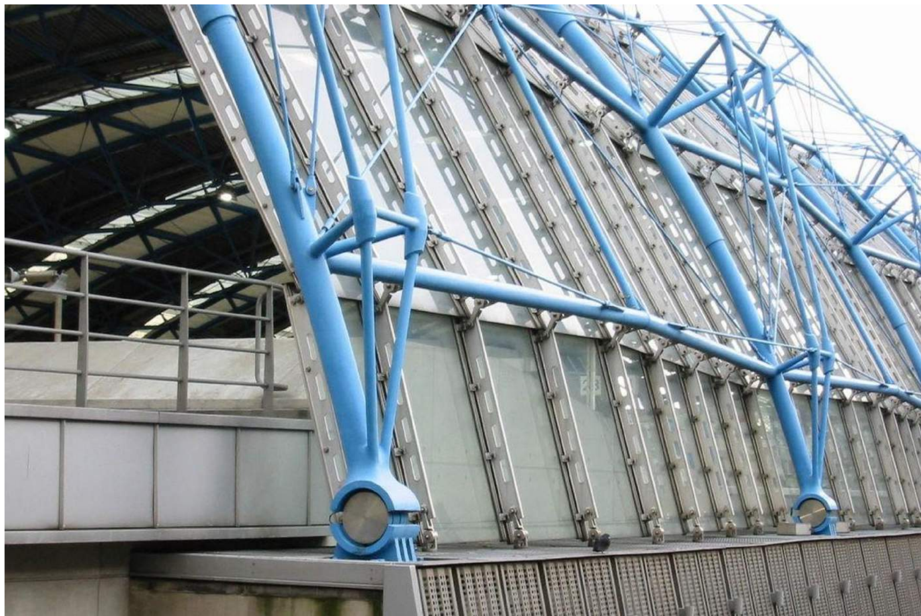
Sir Nicholas Grimshaw (Arch.), Anthony Hunt (Eng.): Waterloo International Terminal, London UK, 1993
