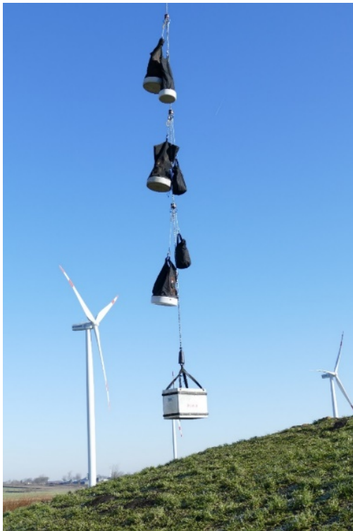
Chain Interlocking Suspension Device on the nacelle chain hoist
