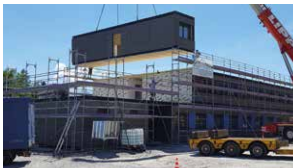
The BI mA is using a modular construction to meet the Federal Police’s rapidly growing need for space.
