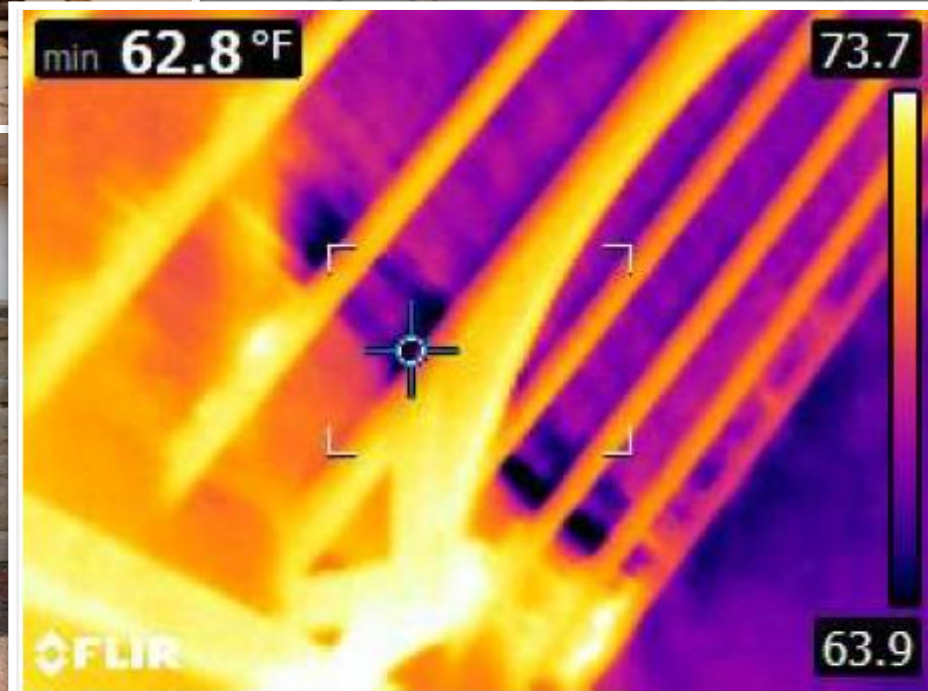
Thermal infrared image of the underside of the roof deck of the main entry. The purple is located directly under the gutter above.
