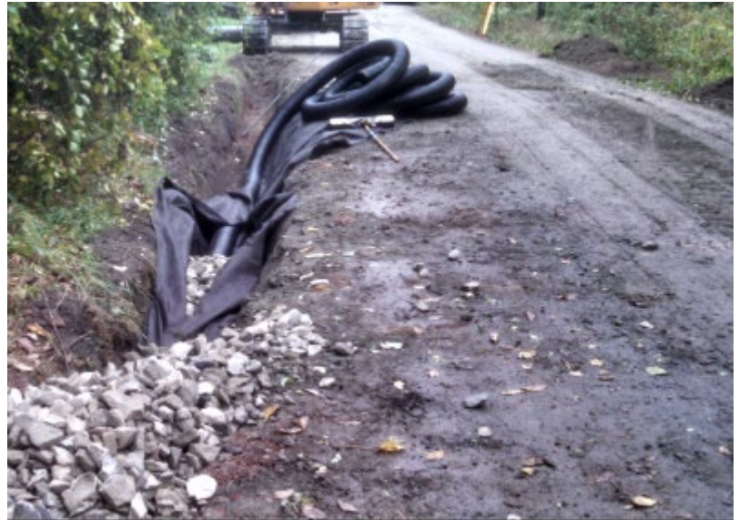
The ditch above was always wet from roadside springs. This underdrain will collect spring flow to keep the roadbed and ditch dry.
