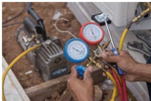
Fig. 4.5.3.10 : Measuring pressure using manifold gate
