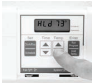
Fig. 4.2.3.3: Checking the functioning of front control panel
