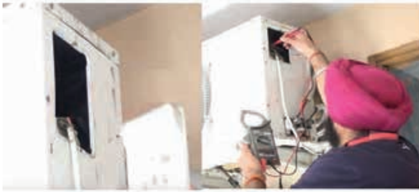
Fig. 4.5.3.9 : Measuring voltage and current
