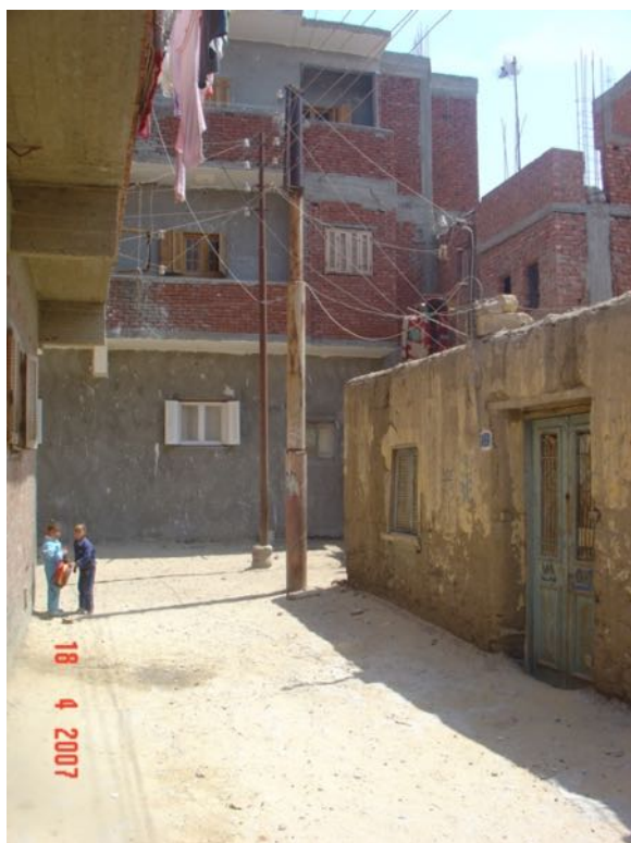
Photo 20: Old Aerial un-insulated Electricity Network
