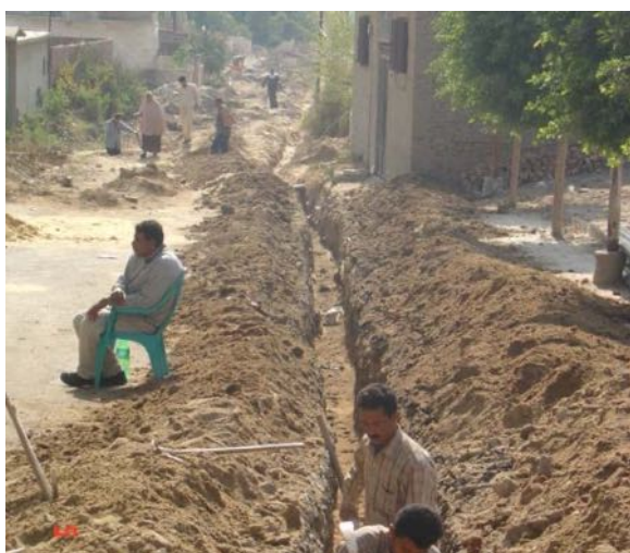
Photo 29: El-Bahtini Sewage Line
