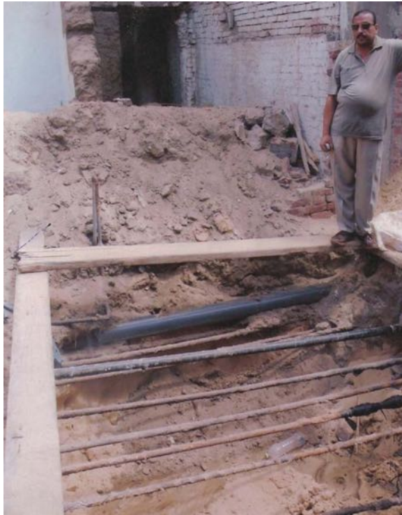
Photo 16: Informal water connections
