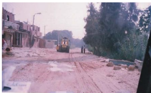
Photo 19: Pavement of El-Hallous Main Road
