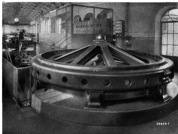
Fig. 1. — Aarau Electricity Works. Two-phase generator Type B 5000/96, 500 kVA, 2000 V, 38.5 cycles, 48 r.p.m., delivered in 1905.
