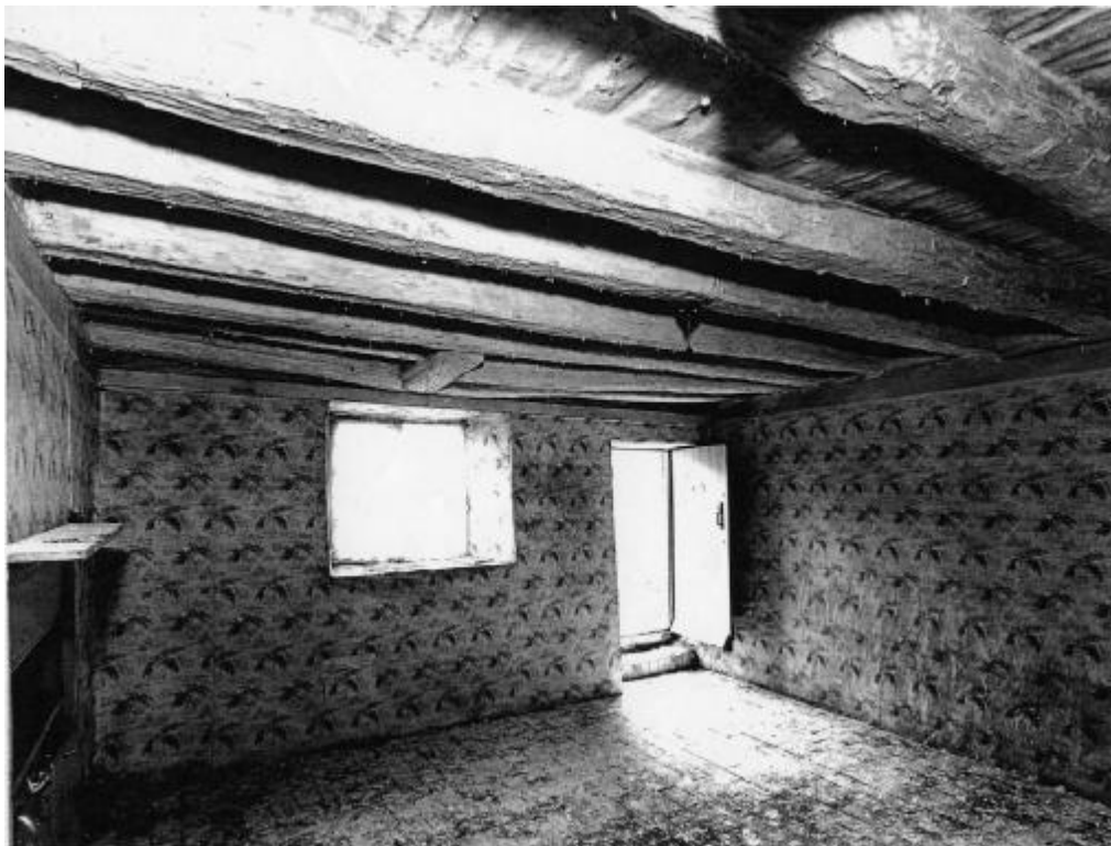
Interior of the same room showing the step down at the entrance Courtesy © Crown Copyright. NMR Ref BB68/2069
