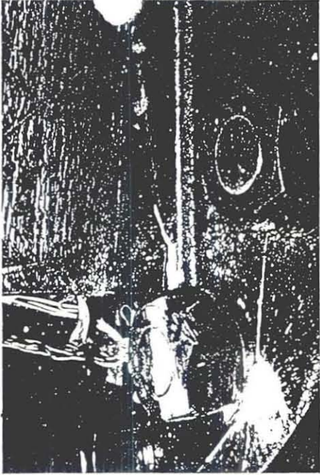
Photo 3 Failure due to Crack of Steel Column near Tension Side of Lower Edge (Type-C)
