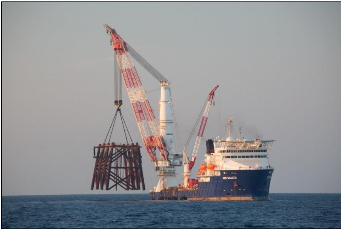
Figure 1.4. Dynamic positioning vessel Nor Goliath lifting the top section of the platform's underwater structure in July 2018. Photo: G.P. Schmahl/NOAA
