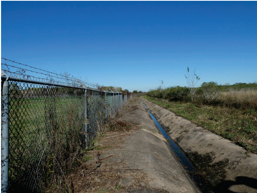
DOP North drainage feature directing surface runoff from drainage roads to Mud Gully
