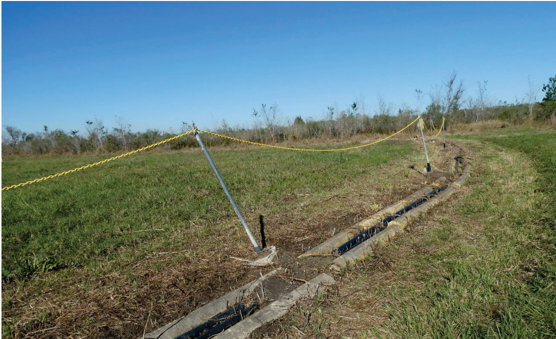
Aboveground groundwater extraction water line across DOP South cover
