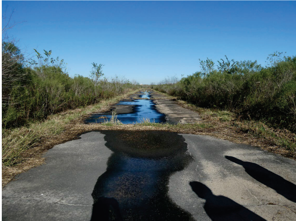
DOP North drainage road, which ultimately drains surface runoff to Mud Gully
