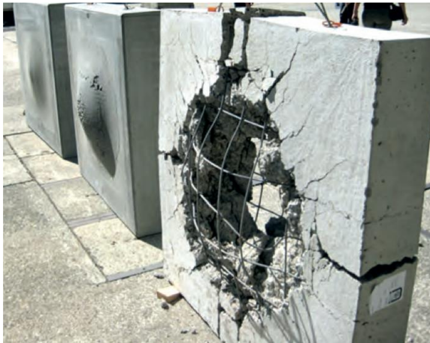
Figure 58: Reinforced concrete slab with punching failure due to explosion
