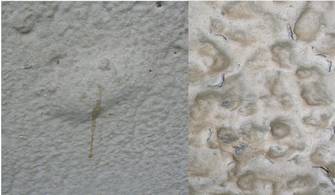
Figure 51 a & b: a) Blistering and delamination of spray-applied membrane, b) Tension cracks in spray-applied membrane
