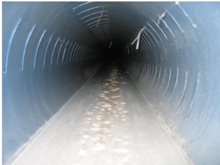
Figure 44: Precipitate in a drainage conduit
