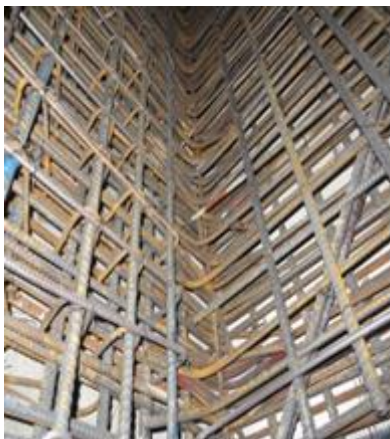
Figure 33: Reinforcing bar congestion
