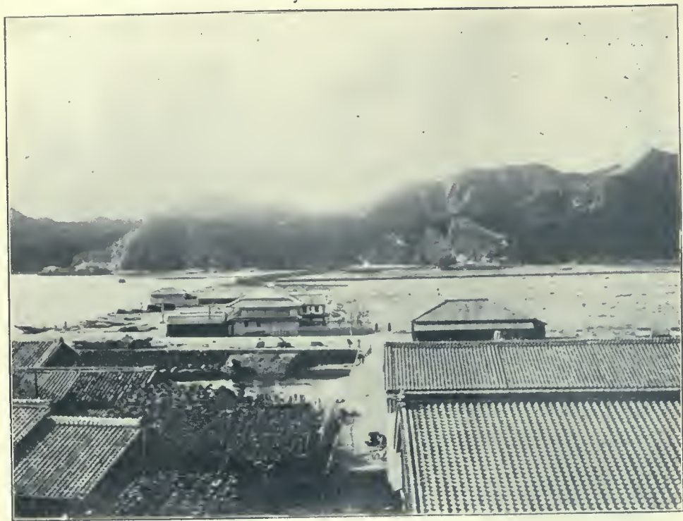
和歌山縣東牟婁郡勝浦村ノ港灣埋立工事 Filling-Up the Harbor of Katsuura Village, Higashi-Muro District, Wakayama Prefecture.
