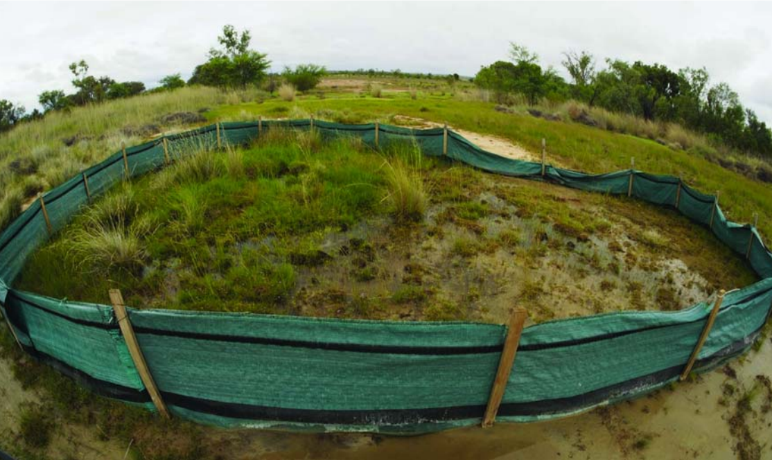
Silt fence installed around a spring containing a relocated population of Blue-eyes at Edgbaston. A.K.
