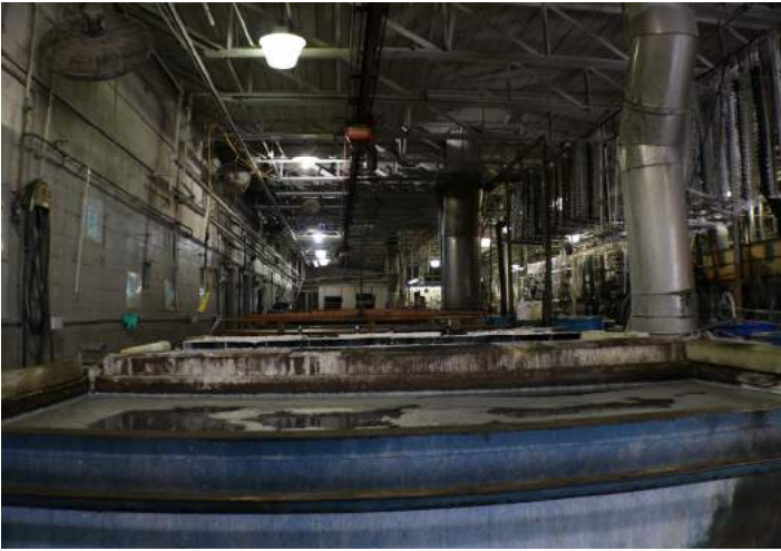
Traditional lighting makes large areas difficult to light.
