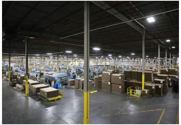
PCG's 522,000 sq ft now clearly lit in every area, promoting employee safety.
