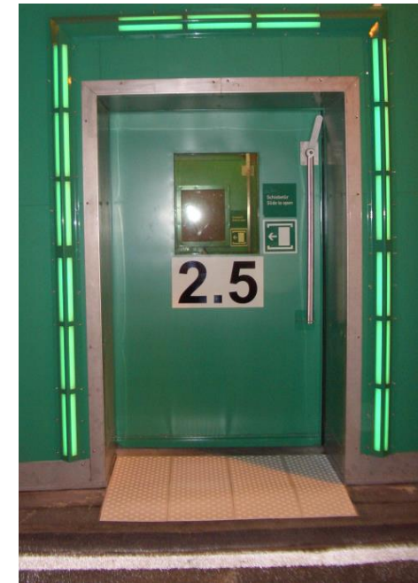
pictograms and text in German+English to indicate the door opening direction + tactile elements for the visually handicapped
