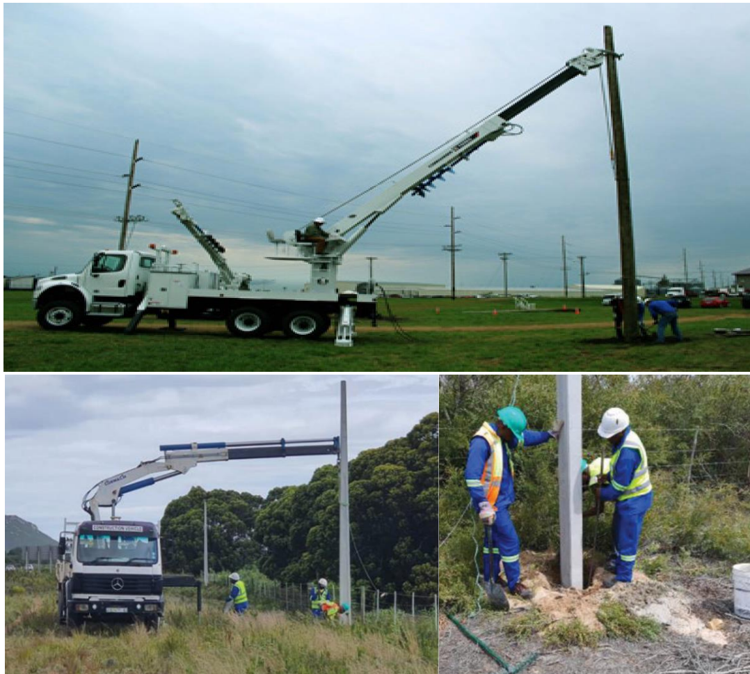
Figure 9: Example of a truck used to plant timber (top) and concrete (bottom) poles.
