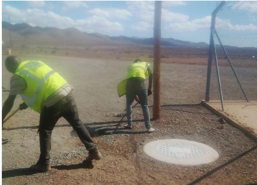
Figure 6: Example of a surface manhole to allow access to the underground fibre optic cable during operations and maintenance.
