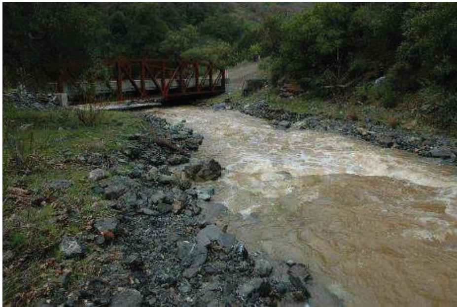
Figure E-9. Flooding Event at Arroyo Mocho
