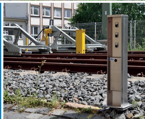
Electric hook-up columns in the daily use
