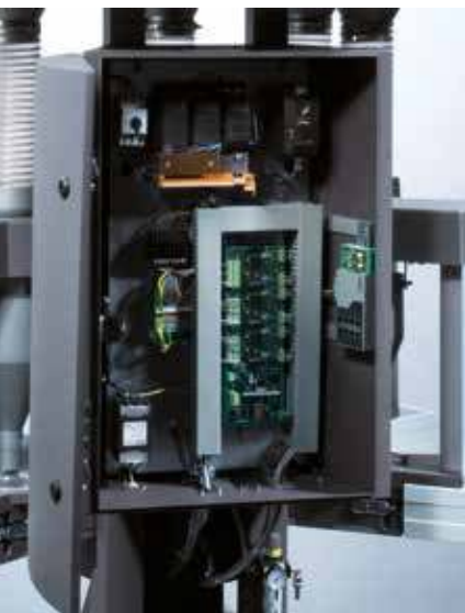
SAVEOMAT switch cabinet
