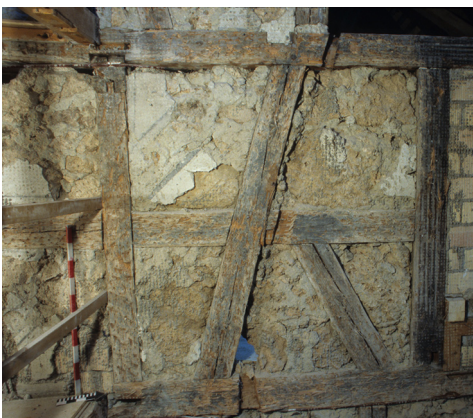
Fig. 9. View of the western wall of the hallway on the second residential floor. Remnants of paint and the closed-off recess for the top step point to the original location of the stairs.
