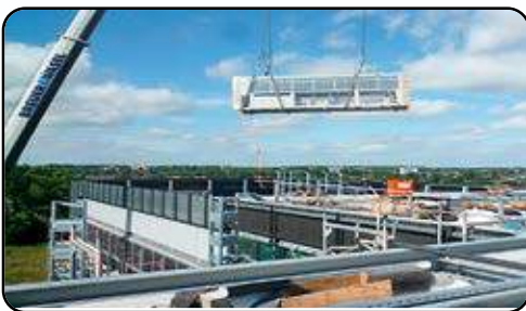
* Chiller installed in Dusseldorf, Germany, 820 kW
