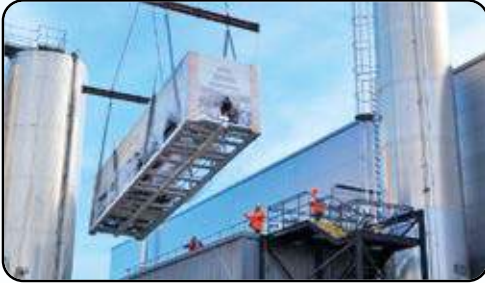
* Chiller installed in UK, 1070 kW
