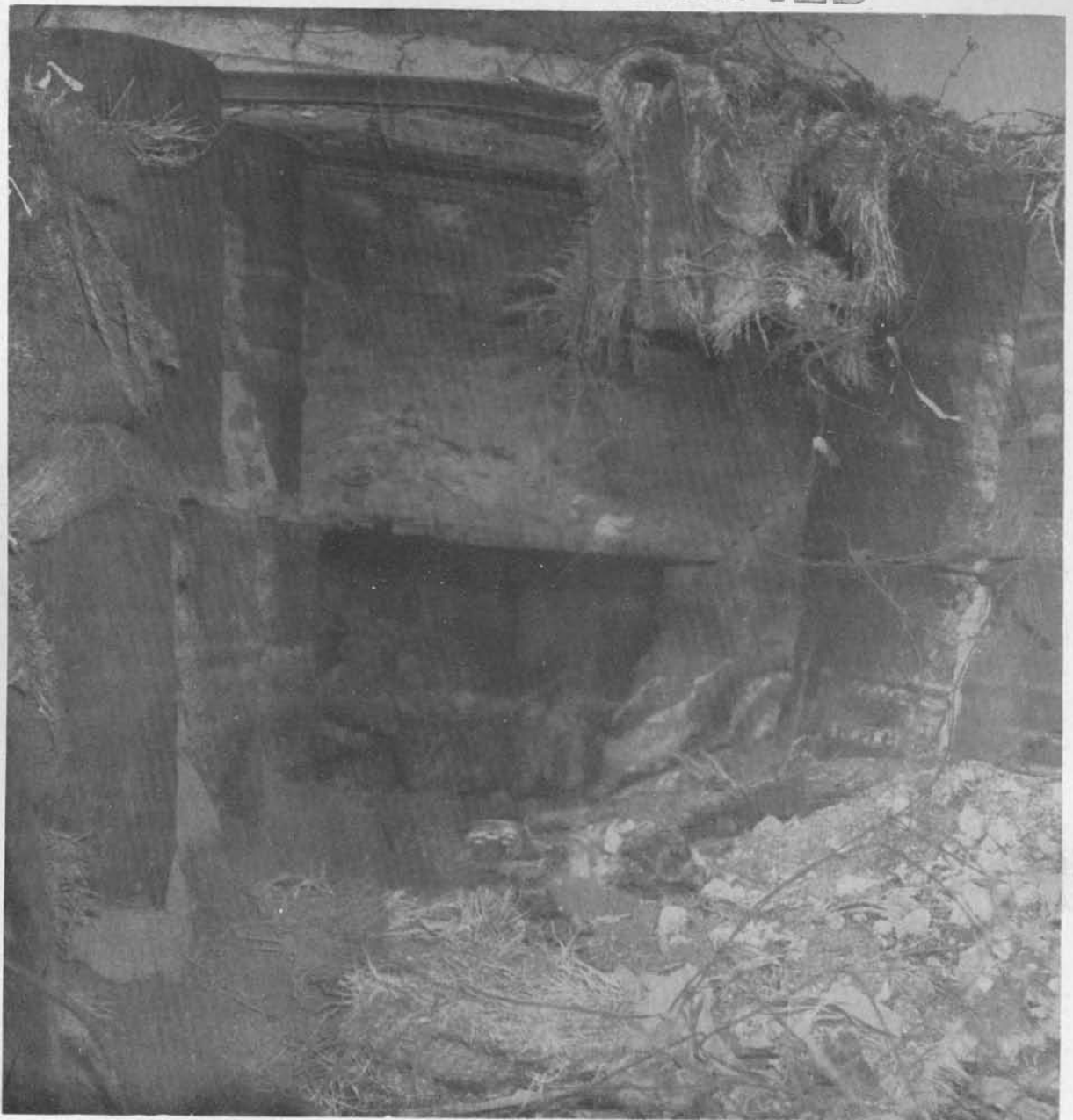
TARGET 119A CLOSEUP OF NORTHEAST FIRING PORT Gun was probably 20 or 40 mm.
