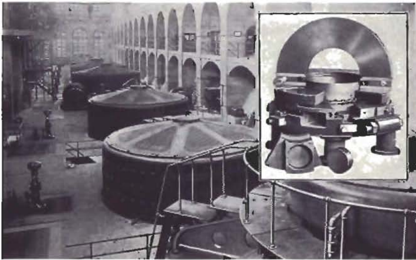
Holtwood Station of the Pennsylvania Water & Power Company. Kingsbury Thrust Bearings are 48 and 56 inches diameter. They are of the separately-adjustable (not equalizing) type. One of them is shown in the inset, with one shoe removed and one-half of split runner turned up on edge.
