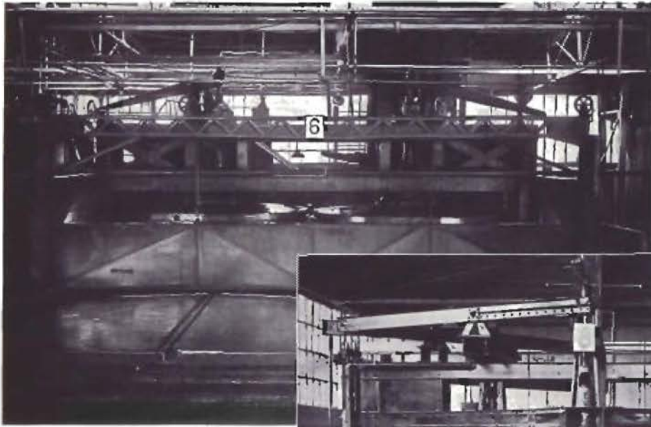
Left and below: Kingsbury Thrust Bearings support the plate glass grinding and polishing machine tables in the Glassmere Plant of the Ford Motor Company.
