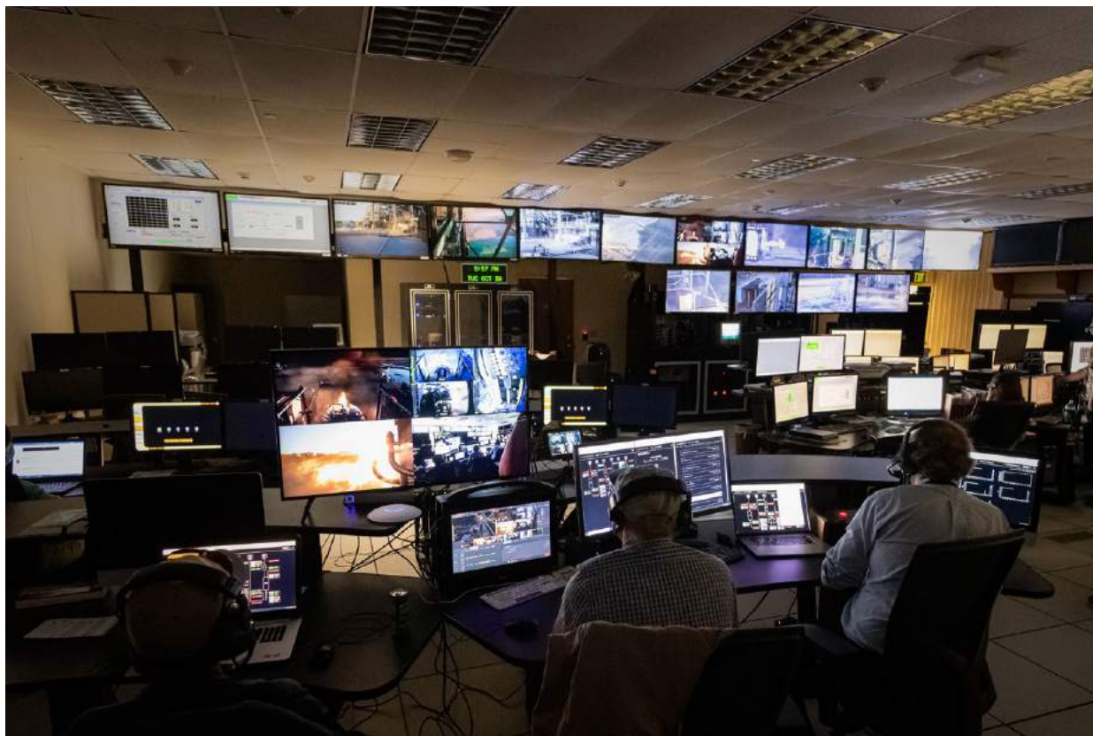
Fig. 11 A control room at NASA's Stennis Space Center during E-2 testing (Courtesy Launcher/John Kraus)
