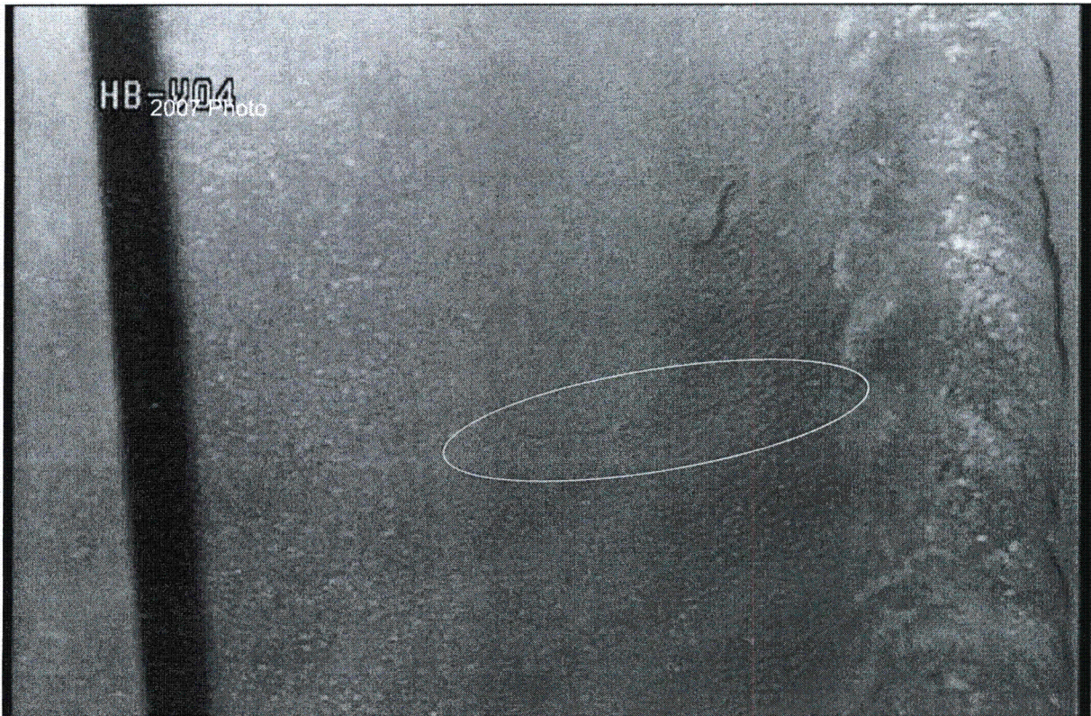
This is a 2007 photo of the 3 rd indication and is a new RFO26 indication.
