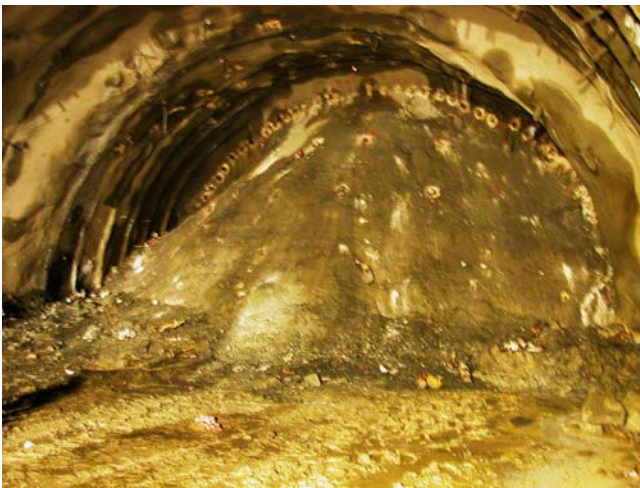
Fig. 20 Appearance of stabilised muckpile at the face. No material has been removed since the collapse and stabilisation has been carried out by the installation of a double forepole umbrella and by grouting
