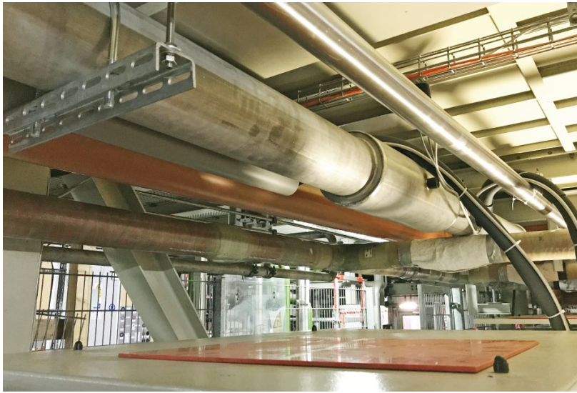
FIG. 9 Superconducting 20 kA Power rail in a chlorine electrolysis plant in Ludwigshafen (Photo: Vision Electric SuperConductors GmbH).
