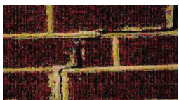
Figure 7.5. Brick Structural Defect
