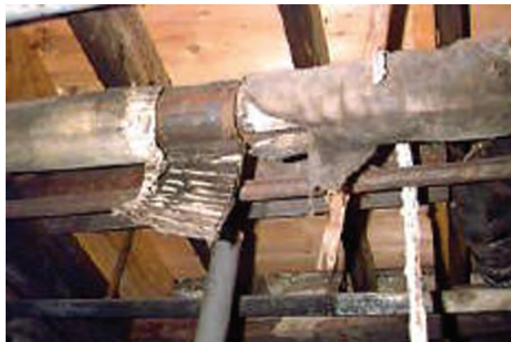
Figure 12.6. Heating Ducts Covered With Asbestos Insulation
