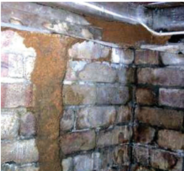
Figure 4.19. Termite Mud Shelter Tube Constructed Over a Brick Foundation [14]
