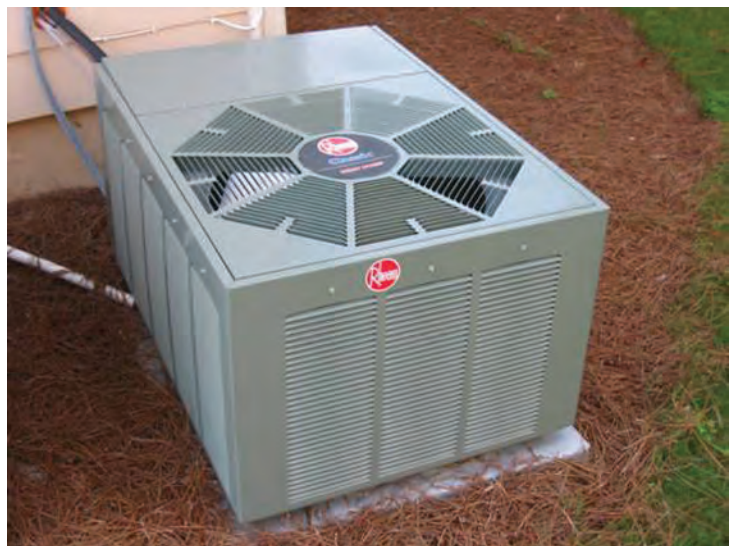
Figure 12.21. External Air-conditioning Condenser Unit
