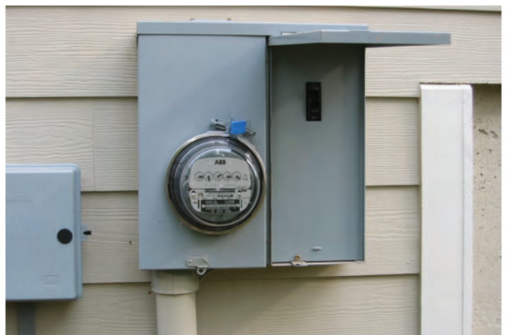
Figure 11.15. External Power Shutoff and Meter
