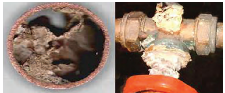
Figure 7.6. Corrosion in Piping Resulting From Galvanic Response
