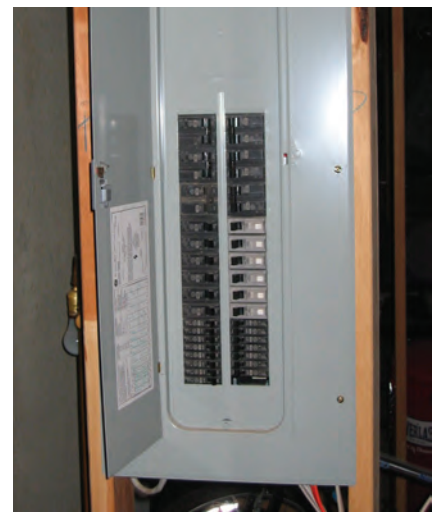
Figure 11.14. 200-Amp Service Box
