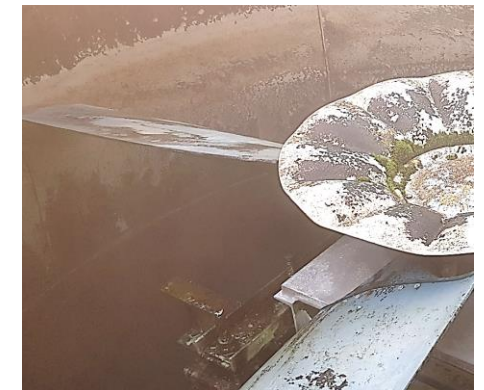
Deposits in the fan area Diffuser
