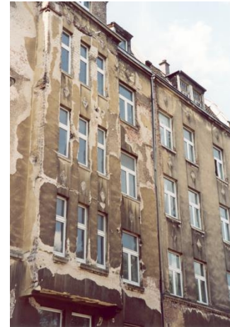
War damages on houses still in 2004
