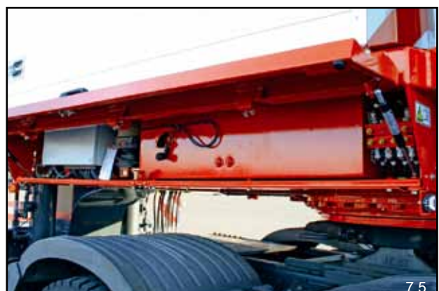
7.5 Full integrated electric PPU within the installation box of the gooseneck
