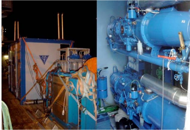
Fig. 6.2.1: Left: Junkers compressor container with pressure reservoir. Right: view inside the compressor container showing two of the four Junkers compressors.
