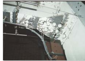
Net section fracture in stem of T-stub
