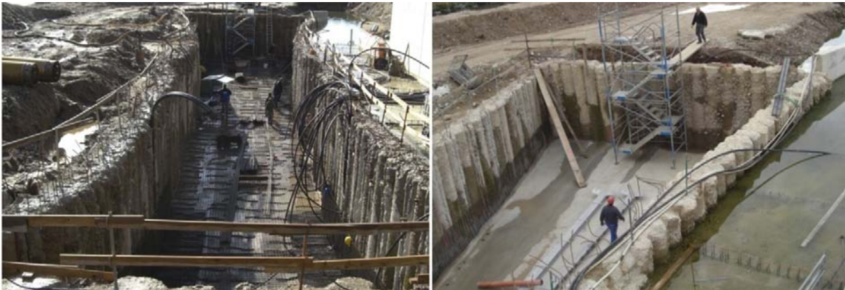
Figure 5: Construction of the trough of the plant made out of secant pile walls
