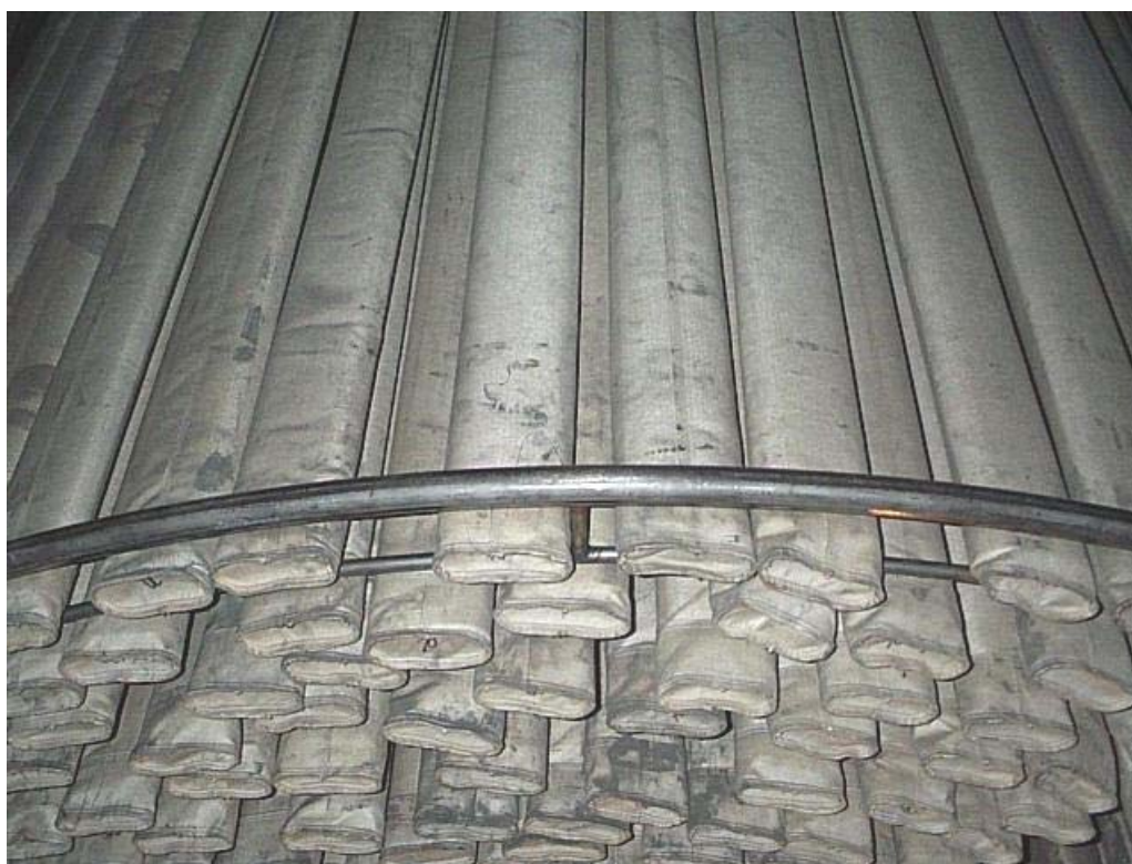
Fig. 5 Photograph of concentric tubular stainless-steel rings installed on Gaston Unit 3 COHPAC baghouse bag bundle 3A10. There were installed to reduce bag movement and bag-to-bag abrasion
