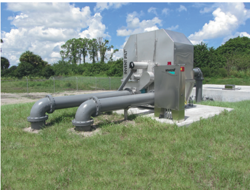
The Invent iFILT-diamond filter at a municipal wastewater treatment plant (source: Invent)
