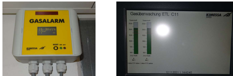
Figure 8: Gas-Alarm Installation in ETL C11. Left: User Panel inside the lab, right: O 2 Concentration display at Lab entry
