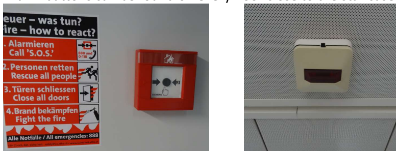
Figure 7: Fire-Alarm button as available close to every staircase and ceiling light indication towards the location of an activated smoke-detector
