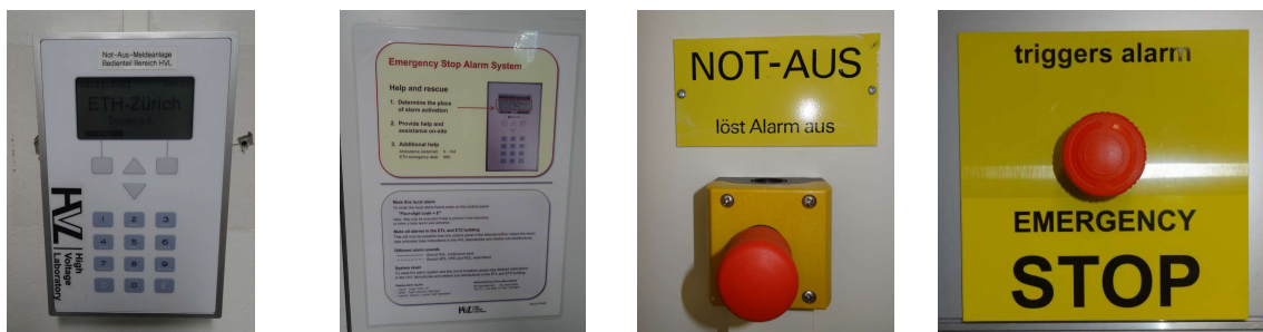
Figure 5: Alarming display panel, manual next to the panel and example of emergency stops labeled in german or english
