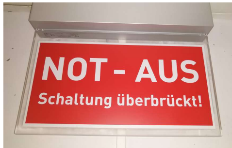
Figure 6: Illuminated warning sign “NOT-AUS Schaltung überbrückt» - indicating works on the electric sub-distribution
