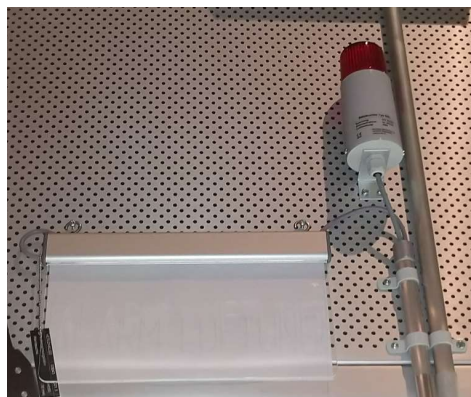
Figure 9: Illuminated ventilation-error sign with associated flash light. warning
