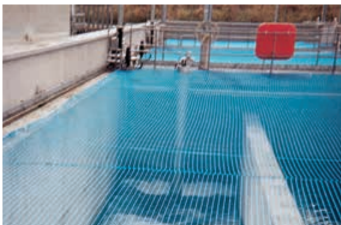
Sewage treatment safety nets
