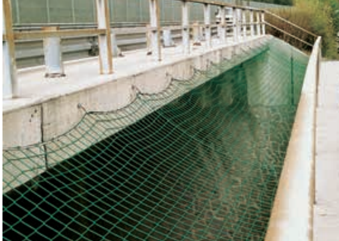
Motorway bridge safety nets
