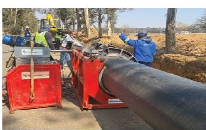
On the 7th September, the A team was out in Sicelo working on the Bulk Water Pipeline.
