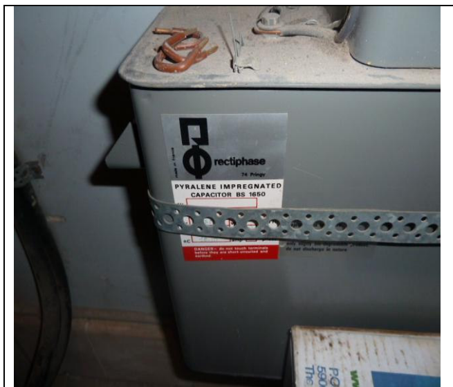
Image 3: Rectiphase Pyralene (PCB) containing capacitor
