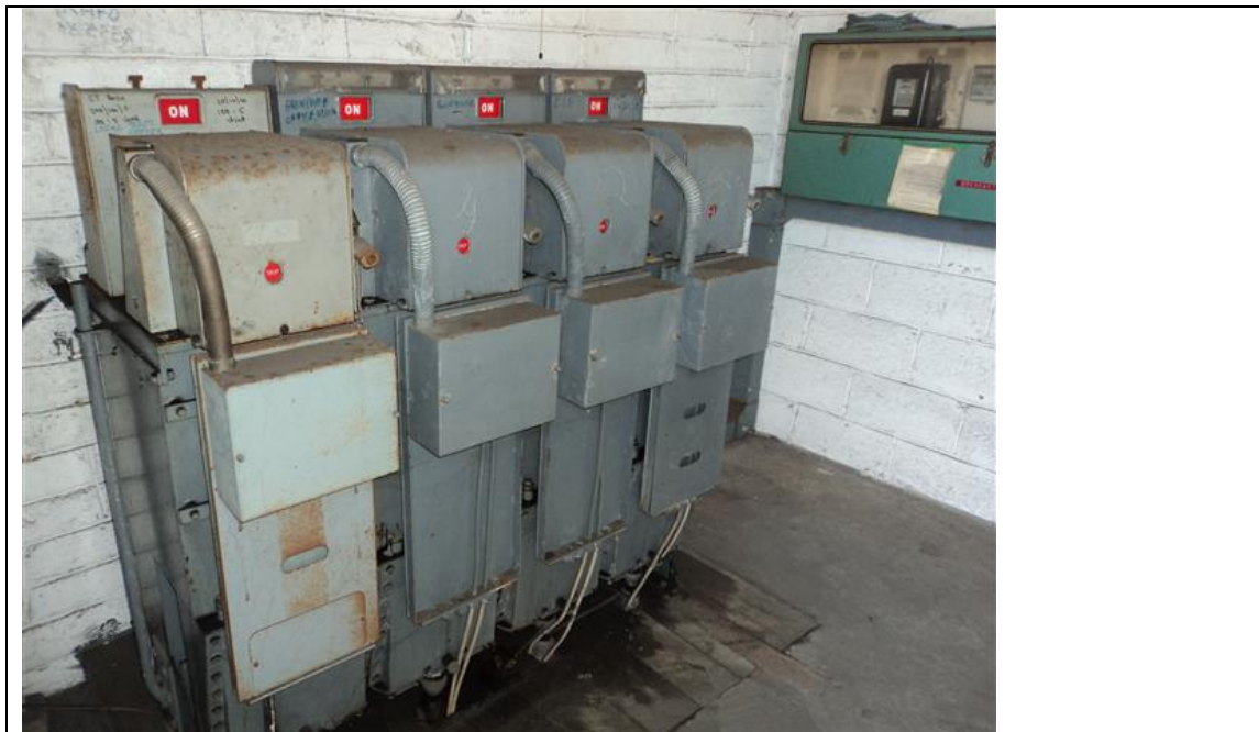
Image 9: Large Industrial Switchgear
