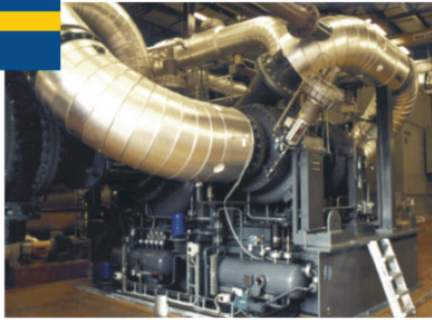
Hammarby, 45 MWq, 3-stage turbo, R134A, heat delivery at 62°C-75°C, source: waste water (7°C-22°C), COP up to 3,48
