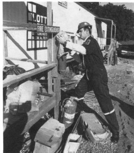
James Helfin of the fire prevention section checks out the fire extinguishers located around the Bldg. 49 construction site.
