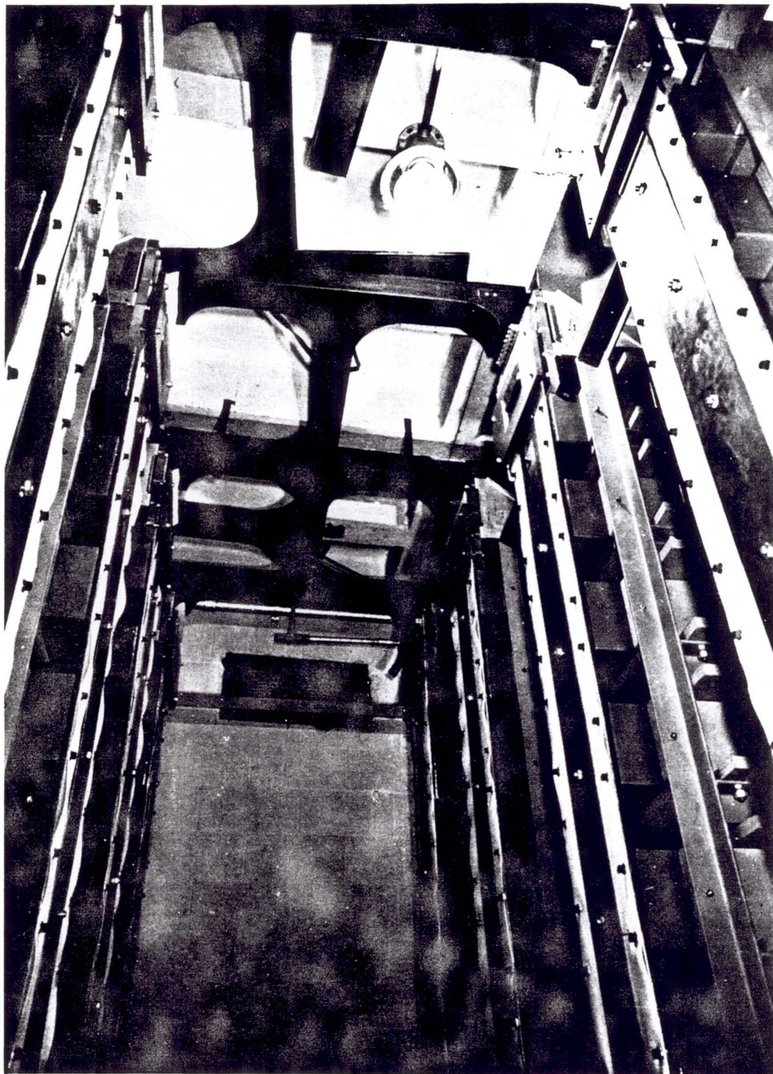
Fig. 31.13 Medusa system capacitor bank during assembly.
