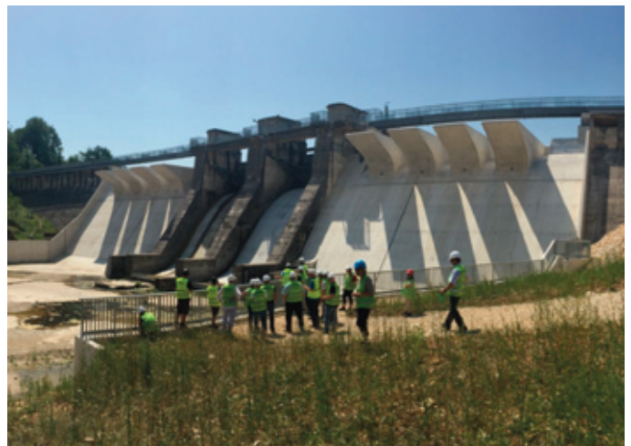
Figure 2. Charmines dam spillway in France with a 23 m wide type-A piano key weir section on both sides of the crest gates (PKW commissioned in 2015). Photo courtesy of EDF.
